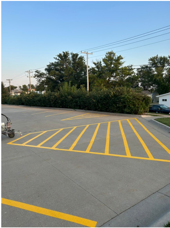
No-Parking Hatching with Equipment
